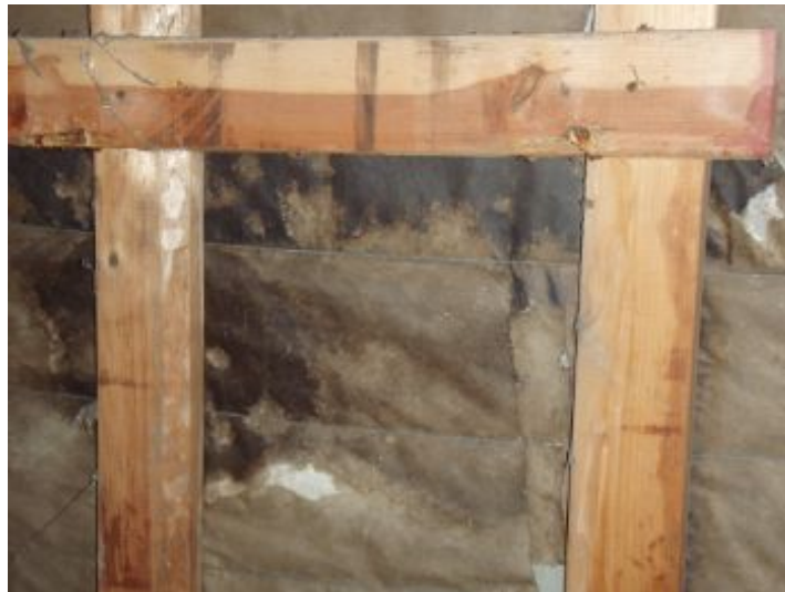
Moister appears to have penetrated the exterior wall at some point.
