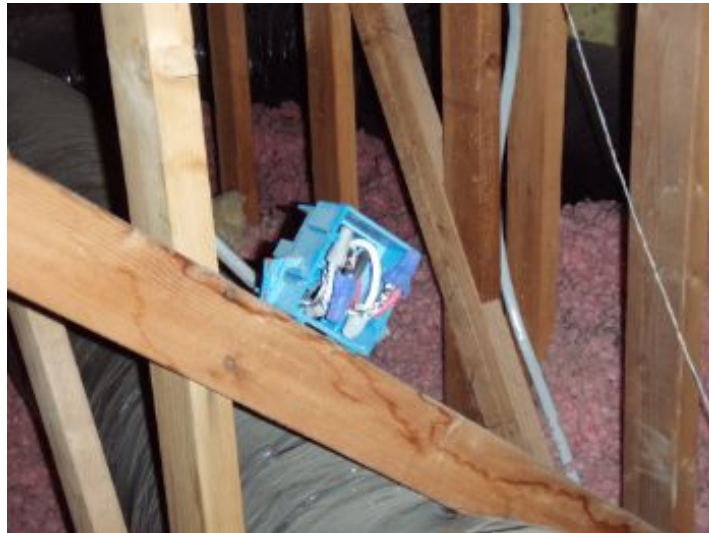
Missing cover plate.
