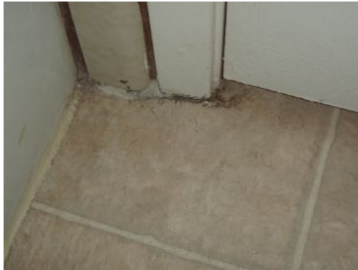
Mold like growth between tub and door.
